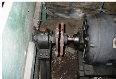
Gt-Ch-Ped blower with no connection to turbine shaft
