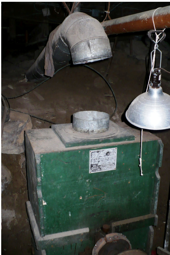
Swell blower motor & turbine connected, but wind line problem
